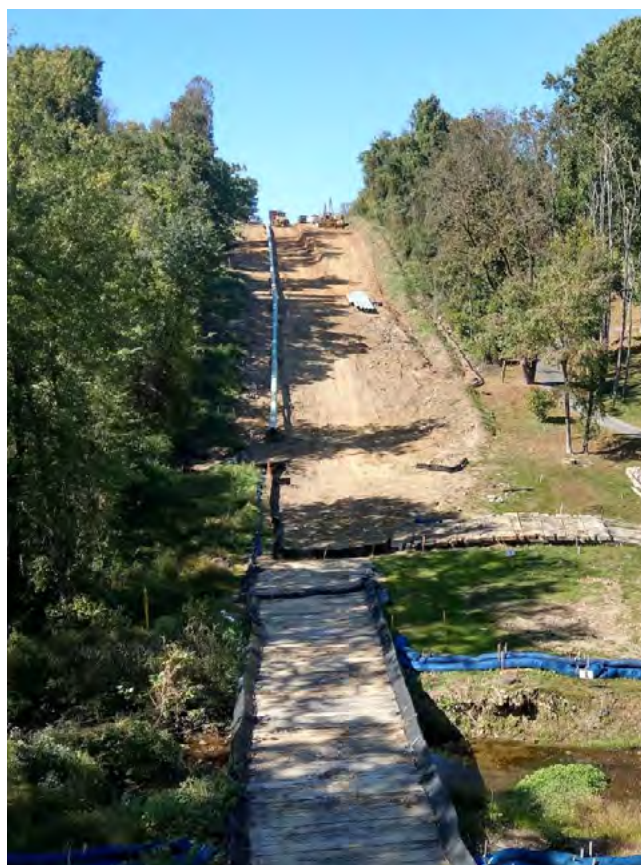
Figure 8.3.2 Example of forest cutting to make way for a new pipeline near Aston, PA, during October 2017. Photo credit: Danielle Kreeger, Partnership for the Delaware Estuary.
