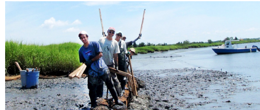
2008 - PDE and Rutgers Haskin Shellfish Research Lab staff installed a living shoreline along eroding marshes of the Maurice River in New Jersey as part of the Delaware Estuary Living Shoreline Initiative. While living shorelines are now an established restoration tactic, they were still an emerging approach at the time and one we are proud to have helped advance since 2008.
